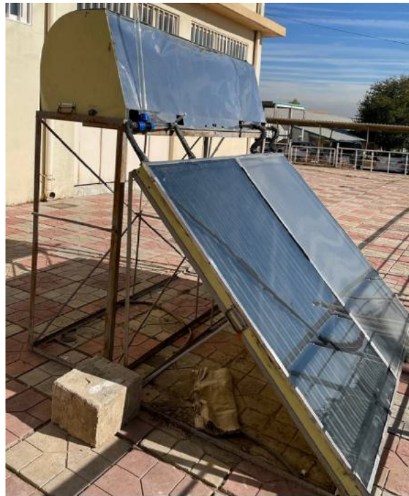
Figure 2. Experimental set-up of the flat plate solar water collector system.
